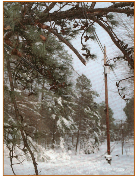
The cost of restoration after hurricanes and the Blizzard of '93 was extensive.
