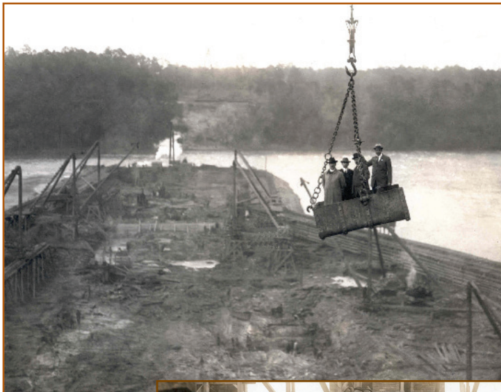
Left to right, James Mitchell, W.W. Freeman, O. G Thurlow and E. A. Yates inspect Lock 12 progress from a construction bucket suspended from an overhead crane, April 18, 1913.
