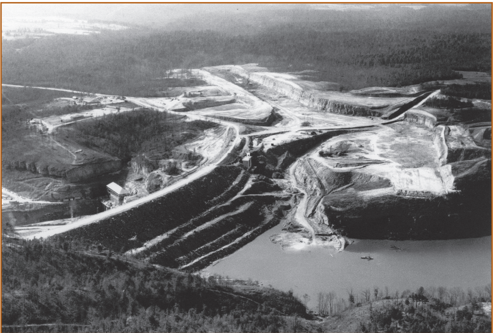
Construction view of Smith Dam looking southwest, January 18, 1961, showing to the center right the emergency spillway to Mills Creek.
