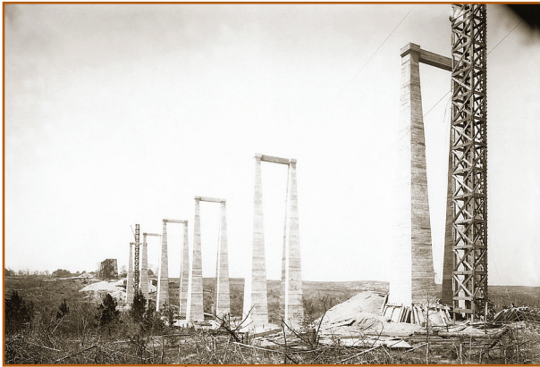
Support pillars for the Kowaliga bridge spans were constructed before the reservoir was filled, April 16, 1926.
